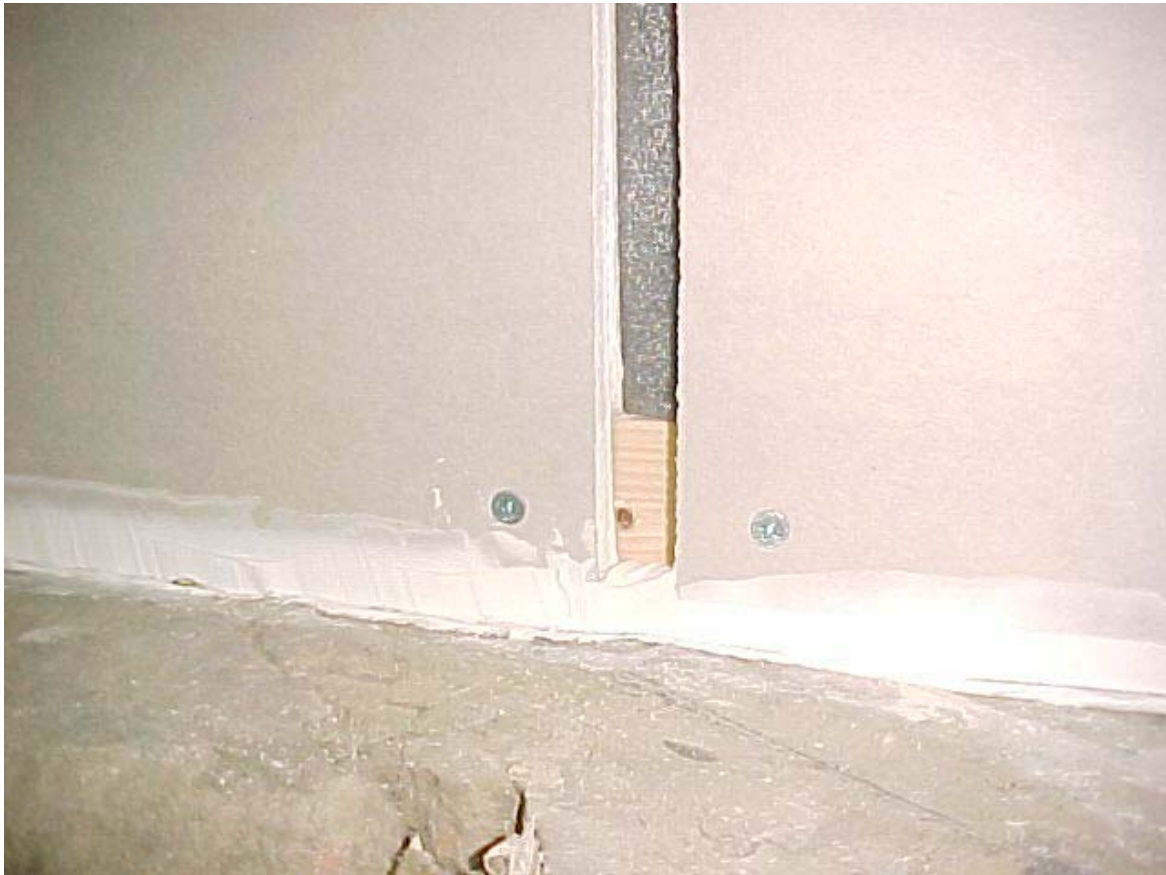
Photograph 3: Partially Unsealed Partition Close-Up
